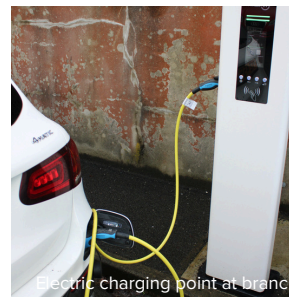
Electric charging point at branch
